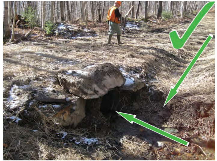
A well placed culvert draining both a direct flow and a ditch line.
