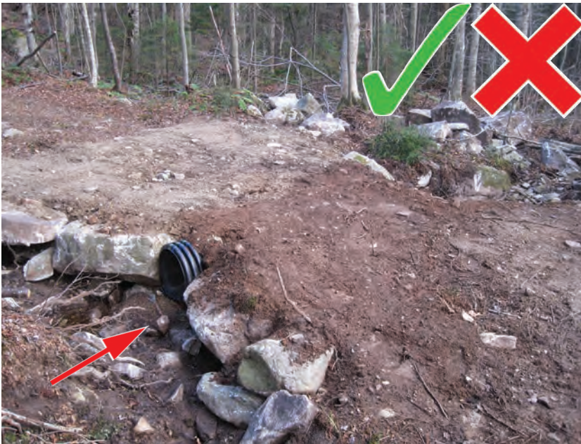
This culvert has a good headwall but is buried too shallow. The tread will quickly erode away exposing the top of the culvert to damage. Additionally, the culvert needs to be set lower to prevent undermining.
