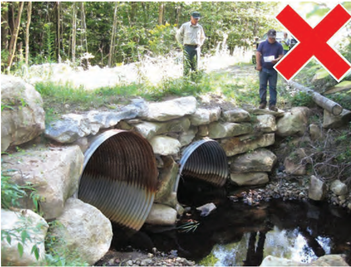
Metal culverts are generally cheaper than plastic ones and their weight can keep the frost from shifting them. Acidic water and soils can quickly rust out the culvert causing it to fail.
