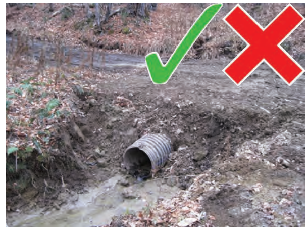
This culvert is set well with ample cover on top. The slope of the fill material is good, but needs seed and mulch or stone to keep it from eroding out over time. Make sure to minimize sediment washing off the construction area.
