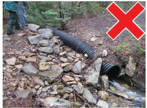
When a culvert is not sized properly, it can blowout causing a lot of damage. It is much cheaper to install a properly sized culvert than to repair a washed out section of trail.
