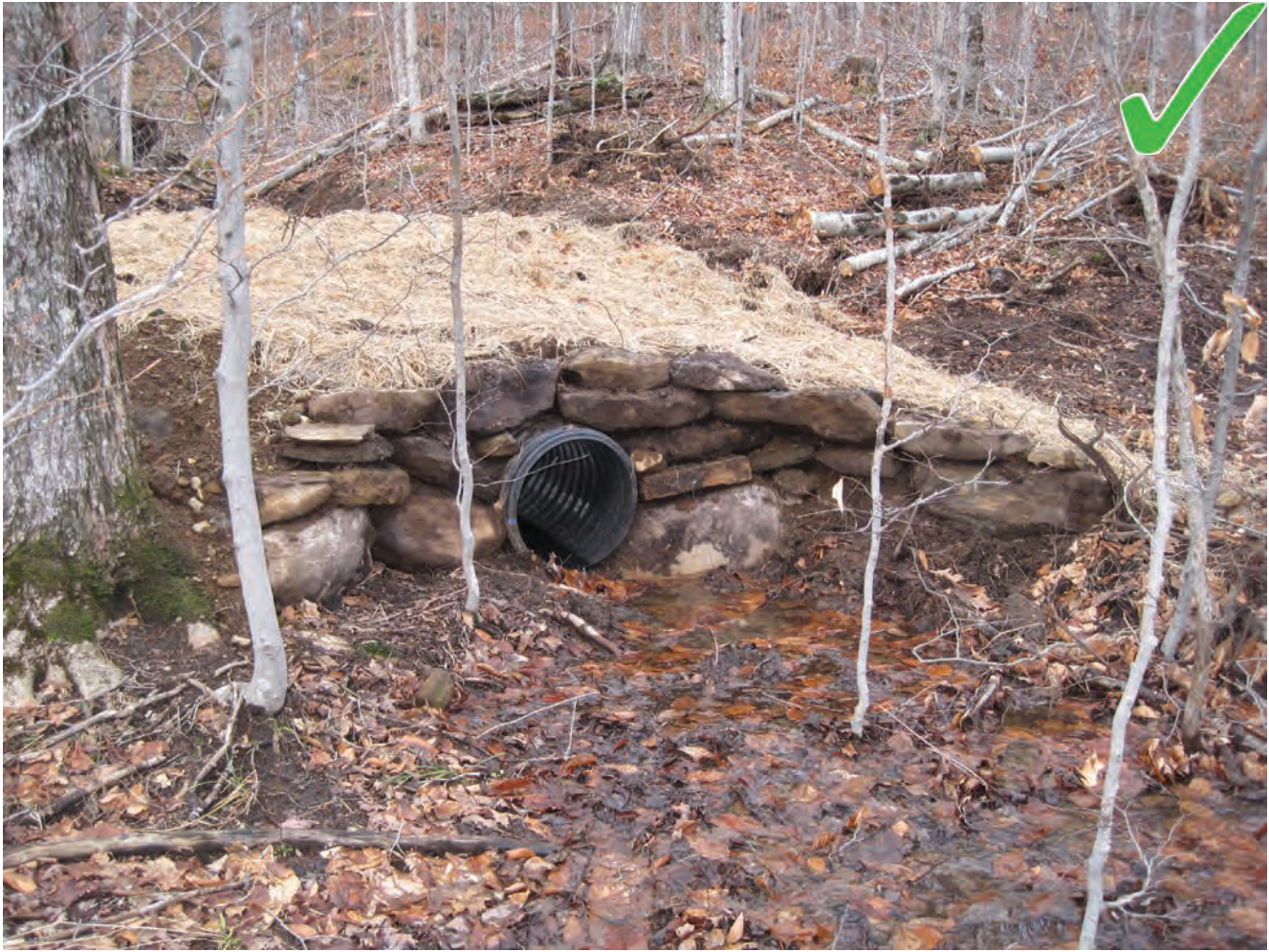
This properly placed culvert has a strong headwall that will keep fill in place and protect the top of the culvert from damage. Seeding and mulching when you are done will further stabilize the soils and prevent erosion. All culverts require annual maintenance ideally in both the spring and fall.
