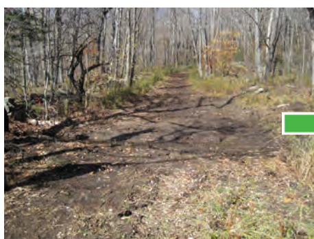
Don't wait to fix erosion in the trail. Once the fine materials wash away, it will be much harder and more expensive to fix. Well built and placed drainage structures will prevent erosion
