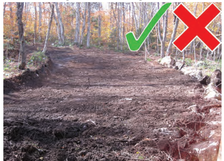
This curve is wide enough to safely accommodate riders. The stones on the outside of the trail could present a hazard to riders who take the corner wide and should be moved.
