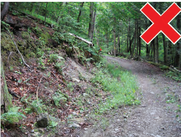
This curve is too narrow and needs to be widened especially considering the reduced sightline from the hillside.
