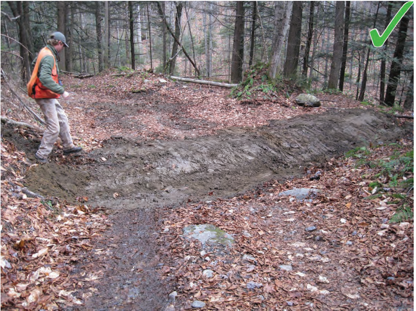
This broad based drain dip is very well built. The shape of the dip is what should be funneling water off the trail via the low point, not the high point acting as a barrier. Drain dips require routine maintenance to function properly. Check them in the spring, fall, and after heavy rain events.
