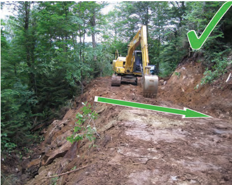
When in-sloping a trail, make sure to include a drainage ditch on the uphill side to control the water flow. Remember to seed and mulch exposed soils when finished.
