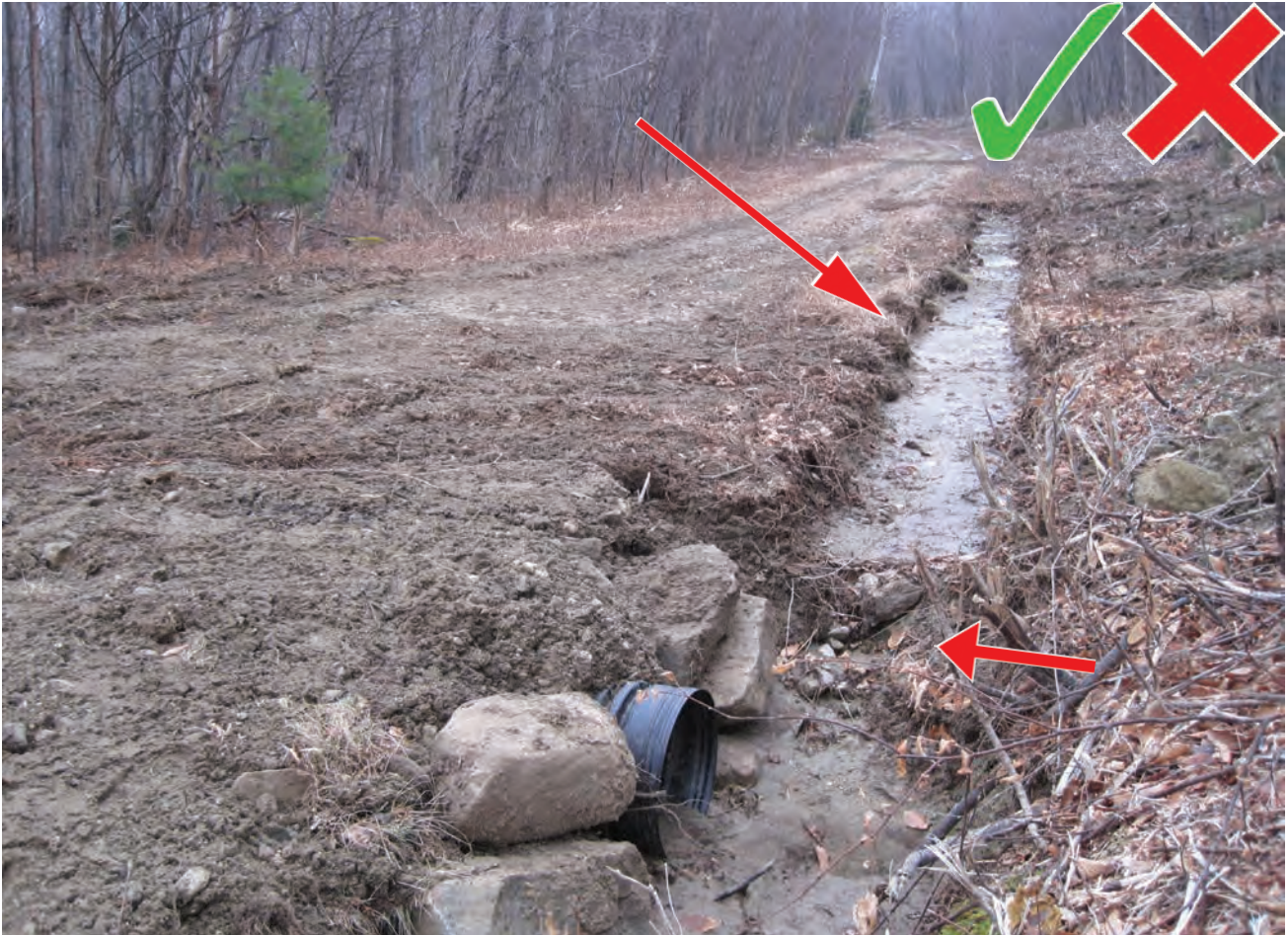
This is a good example of turn-piking. Turn-piking is the process of removing soil material from ditches in low, wet areas and using it to raise the elevation of the tread. Ditches will generally be on both sides of the elevated tread. Water is distributed with a series of cross-drains which are usually culverts but can be drain dips as well. In this example, the ditch could be wider and need to have the sides reshaped. The culvert header has collapsed a bit too. Remember that ditches require regular maintenance to work properly. Make sure to remove any material that has built up to avoid damage to the trail.
