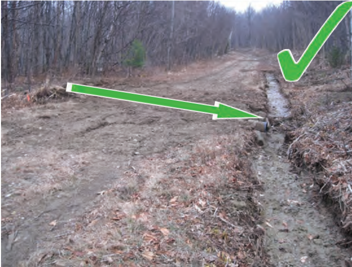
Consistent grades make for an easy to groom, enjoyable to ride trail. Avoid unevenness or abrupt grade changes.
