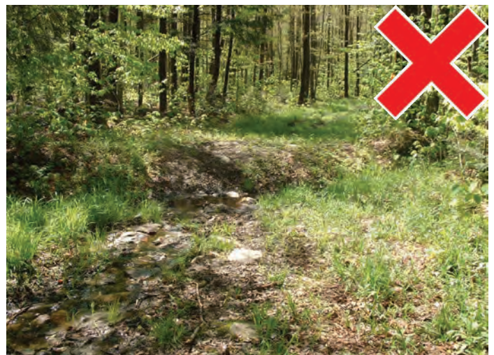
This drain dip is too large and will act as a barricade for trail riders and grooming equipment.
